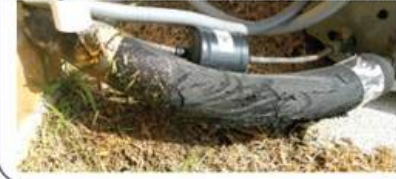
Damaged Insulation from landscape maintenance
